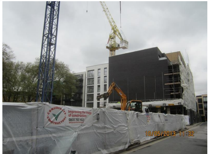
Orchard Building looking east from Pear Tree Street during construction (prior to construction of frontage building)
